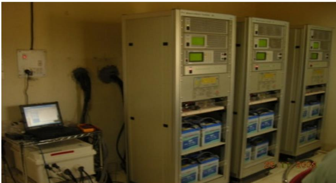
Figure 3.14 Three I-V Scanners, one for each technologies to measure I-V measurements
