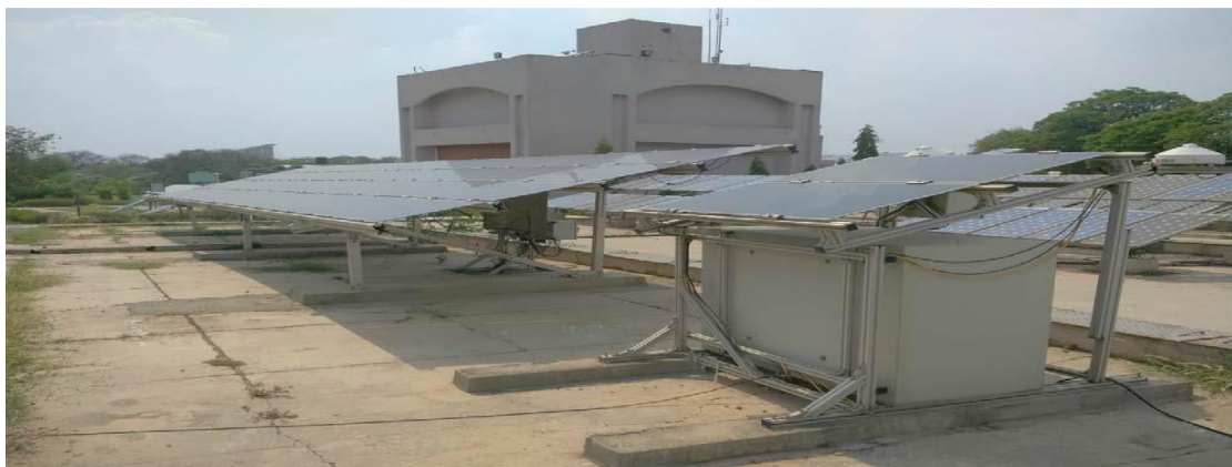
Figure. 4.2 3.2 kWp PV system with reference PV module and Pyranometer
