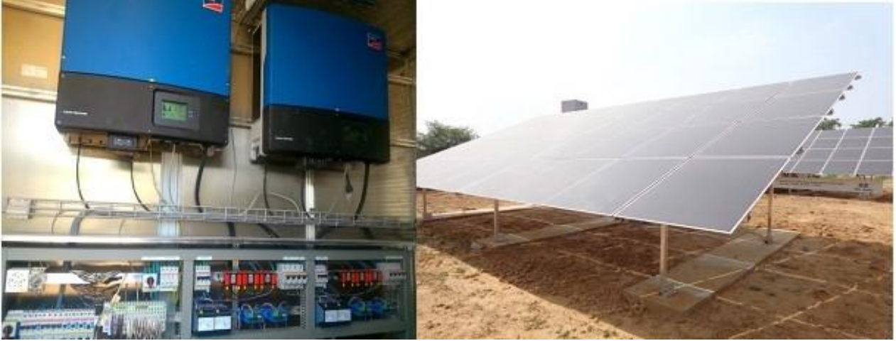
Figure. 4.3 8.64 kWp PV Micromorph Power Plant Along With Control Room
