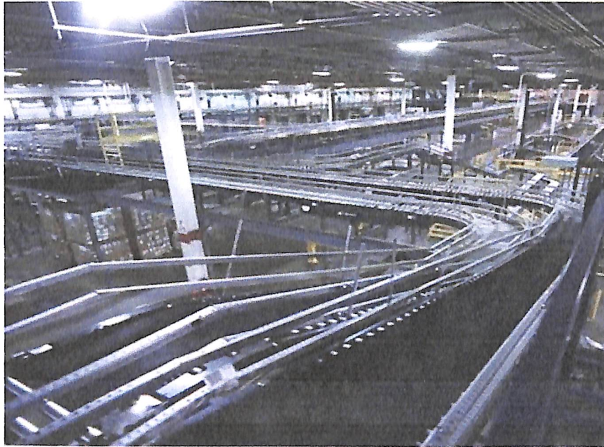
Figure 20: Conveyor System and Carousels
