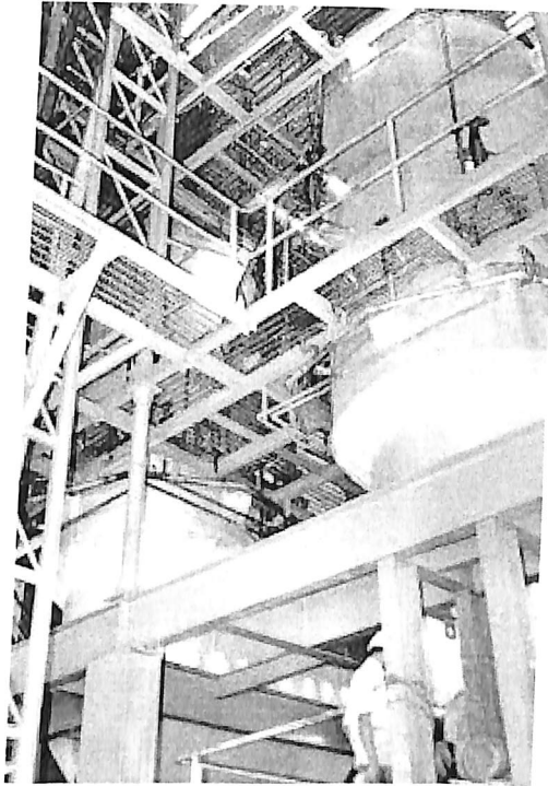
Figure 11: The reactors at Arashi Hi-Tech Biopower Ltd at Sultanpet, near Coimbatore.
