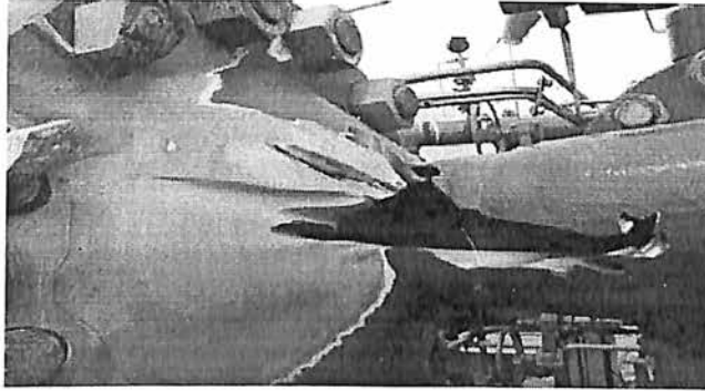
Figure 1.2 Erosion damage to pipes
