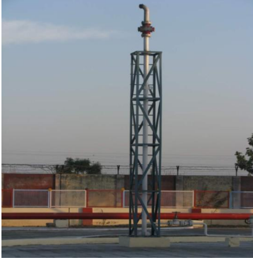
Fig A-6: A Typical LPG Flaring System in a Pumping Station
