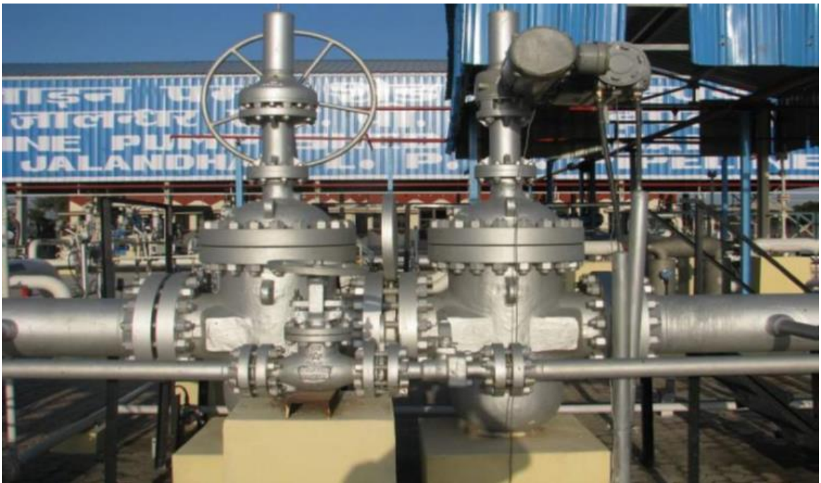
Fig A-5: LPG Station Valves
