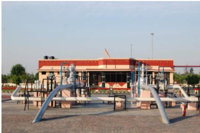
Fig A-7: A Typical LPG Pipe Station Control Room
