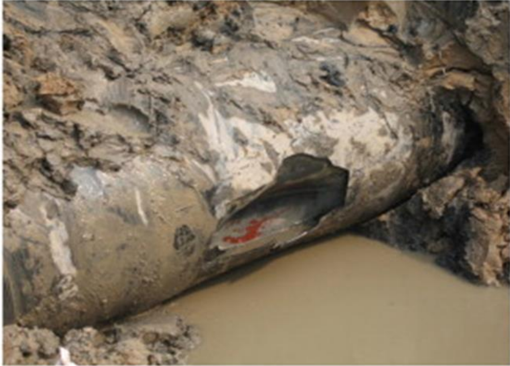
Fig A-9: A Typical Pipeline Damage Due to third Party Activity
