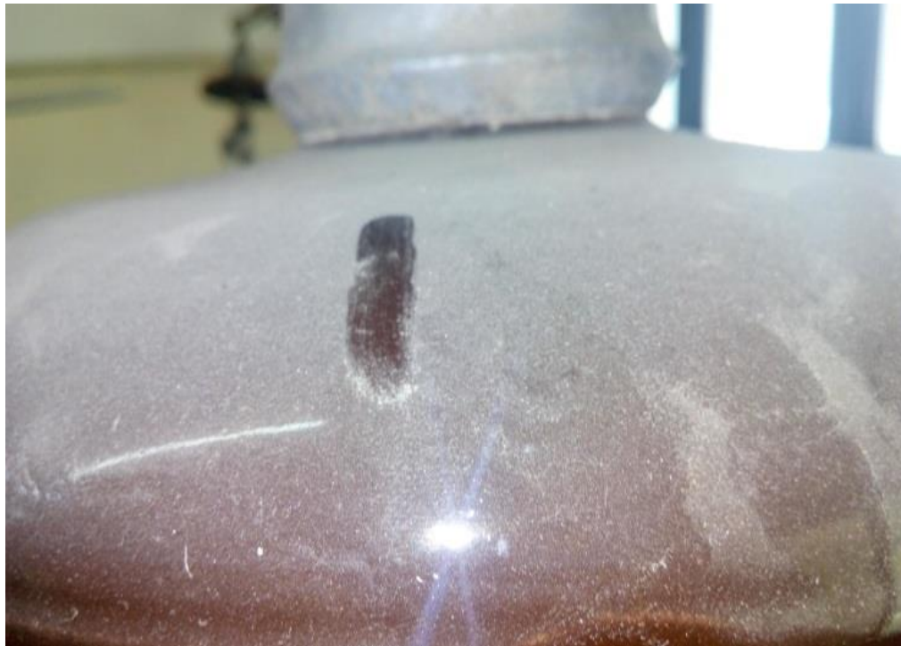
Figure 5-5: Uncoated post insulator with formation of dust layer.
