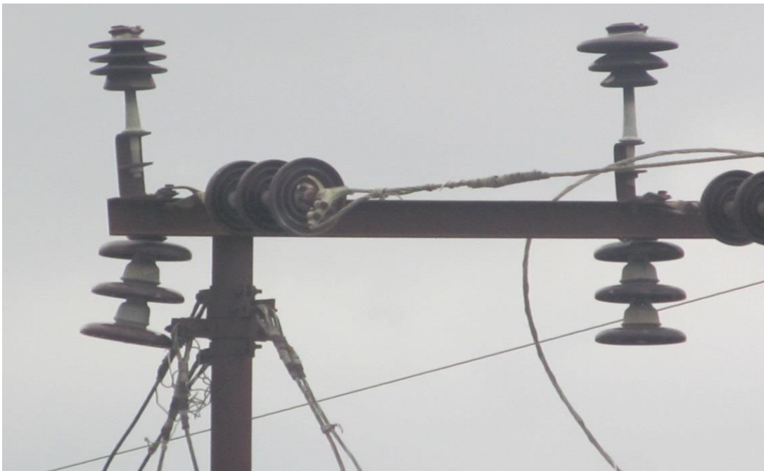
Figure 5-3: Coated and uncoated post insulator was kept at dead end electric pole of 33kV hot line.
