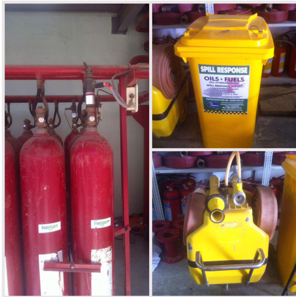
FIGURE 12 FIRE FIGHTING EQUIPMENTS AT VGT
