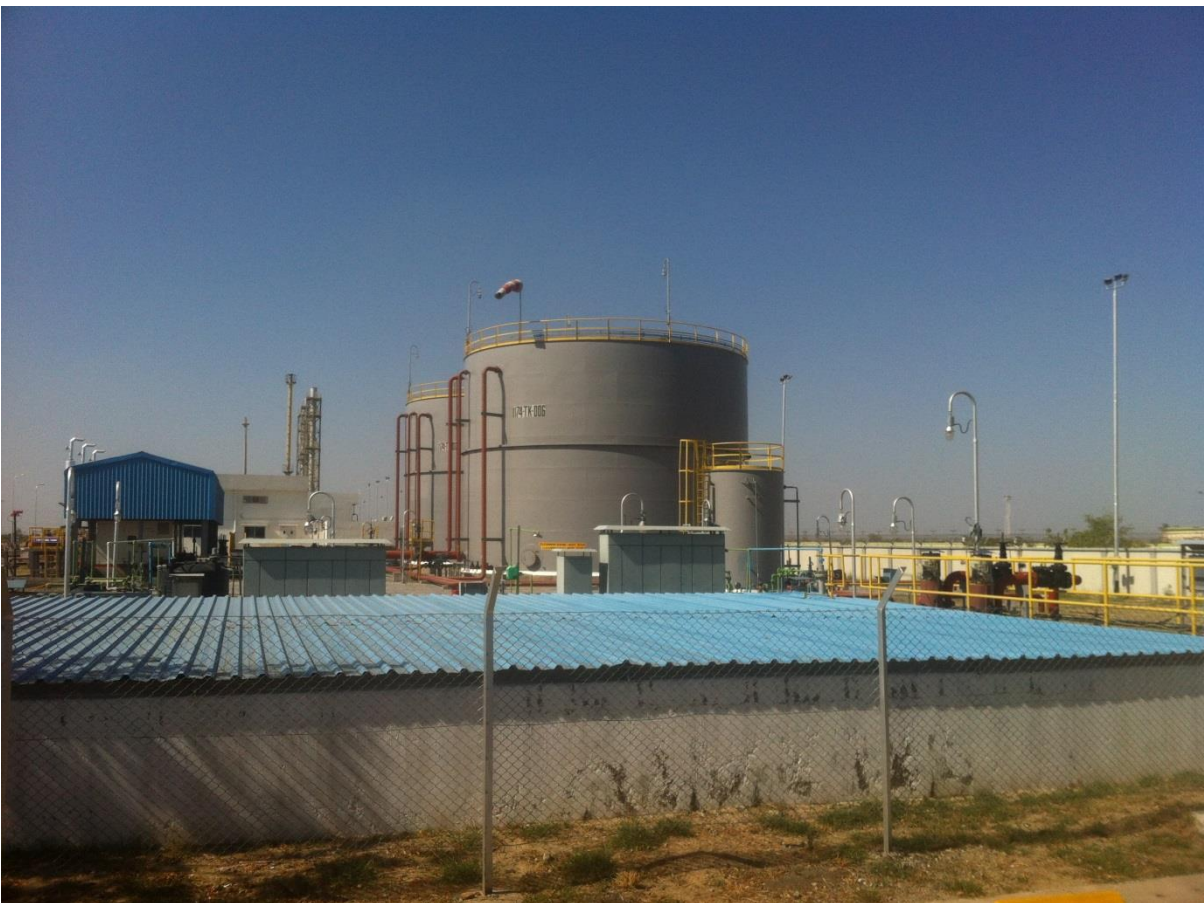
FIGURE 13 WATER TANKS AT VGT
