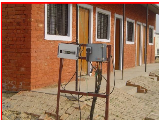
P-35: Improper electrical board
