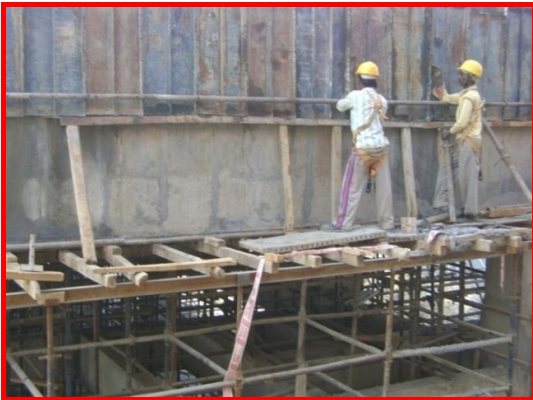
P-21: Unsafe Working Platform
