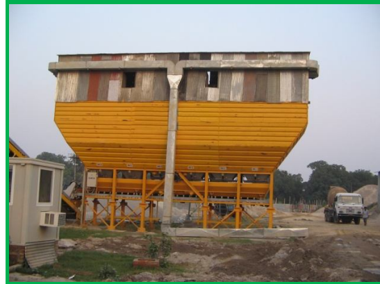
P-2: Enclosed Batching Plant Materials Bin
