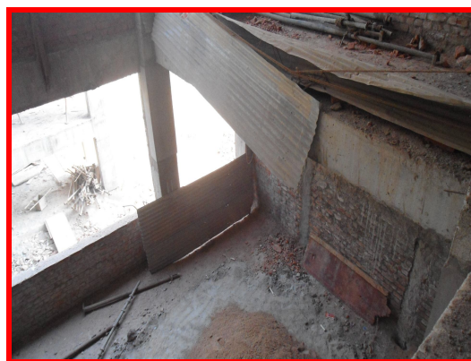
P-30: Hanging unsafe GI sheet
