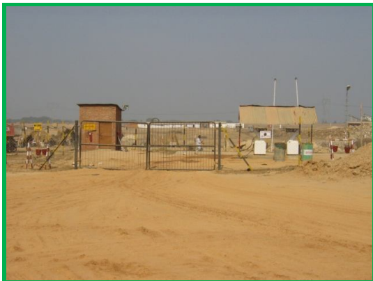
P-11: Safety Arrangement at Site Petrol Pump
