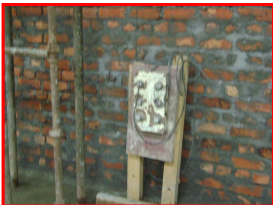
P-29: Unsafely electric board
