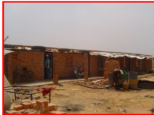
P-32: Unhygienic condition of labour camp
