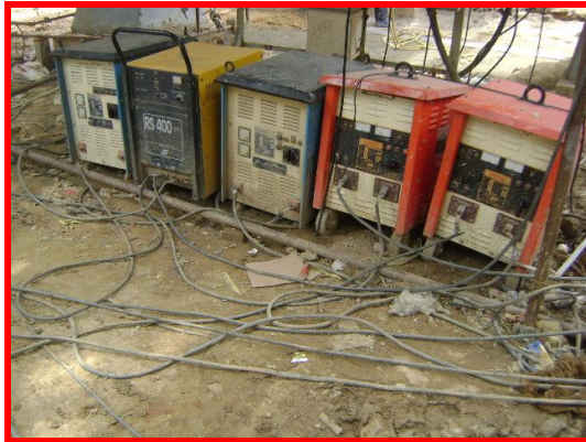
P-20: Haphazard electrical cable
