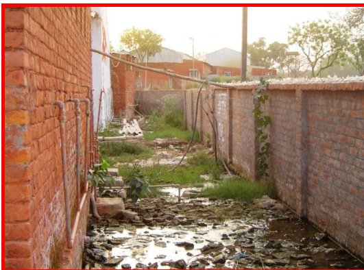
P-33: No Proper drainage system
