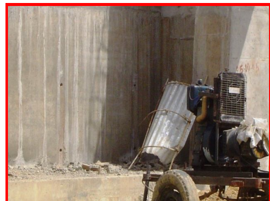
P-36: Unsafe temporary DG set
