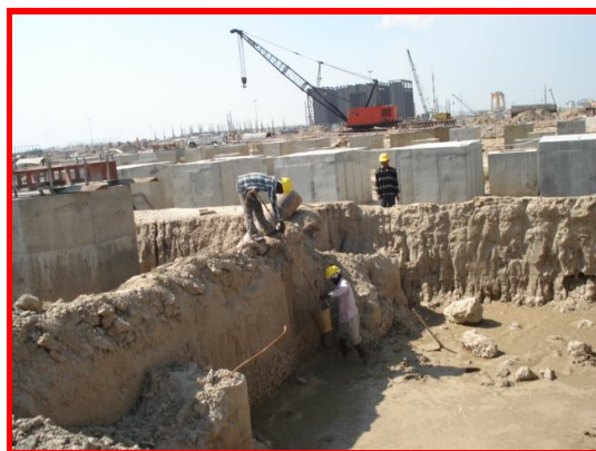
P-24: Unsafe earth excavation
