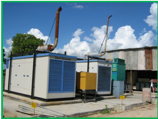
P-3: Stack Height of DG set
