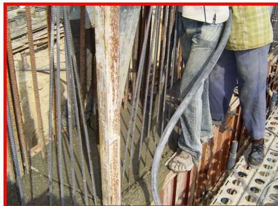
P-34: Unsafe platform & without gum-boot
