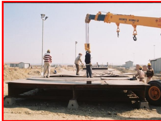
P-28: Unsafe sling and without safety latch in hydra
