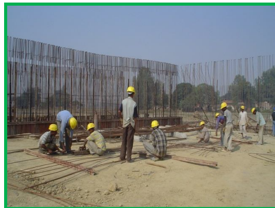
P-6 : Housekeeping and use of PPE by workers
