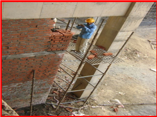
P-25: Unsafe platform & without safety Belt
